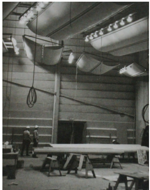
Construction workers lay the original beams of old hardwood on the stage in the spring of 1974.
